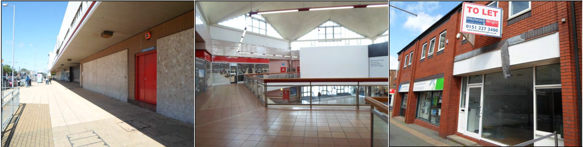
Photograph (left): Boarded frontage to the Strand Shopping Centre on Washington Parade
